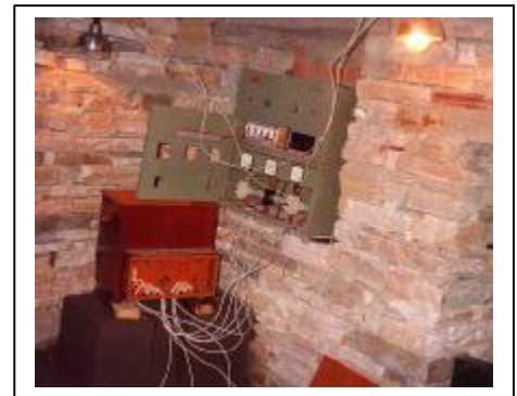
Electronic Load Controller
