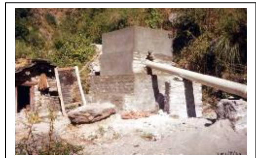
Forebay Tank with Penstock
